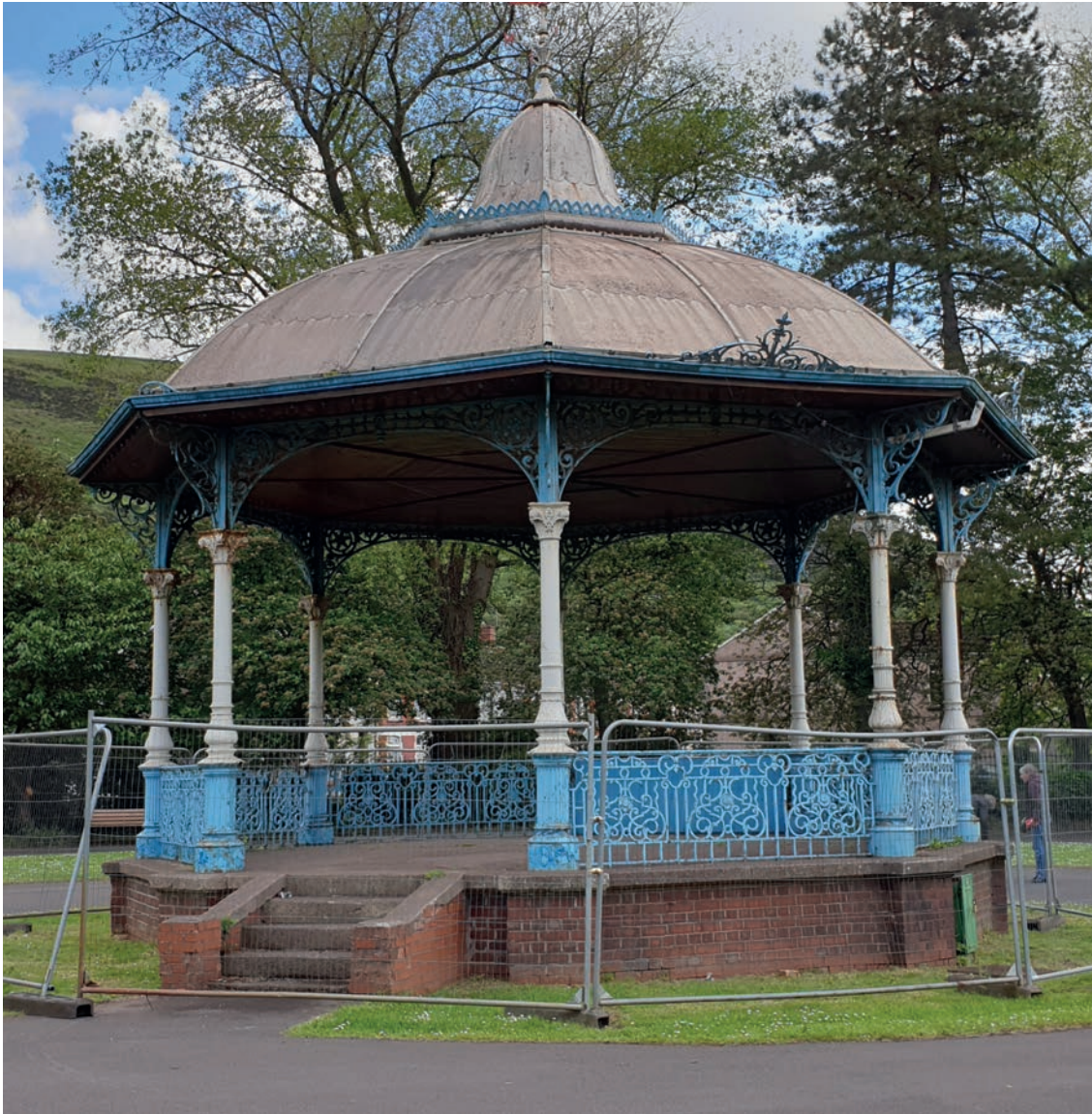
The Bandstand in Talbot Memorial Park in need for maintenance and repair.
